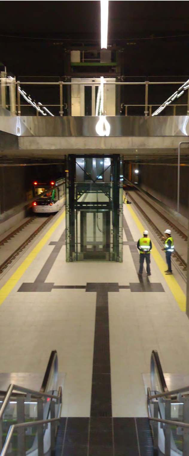
Malaga Metro installations
